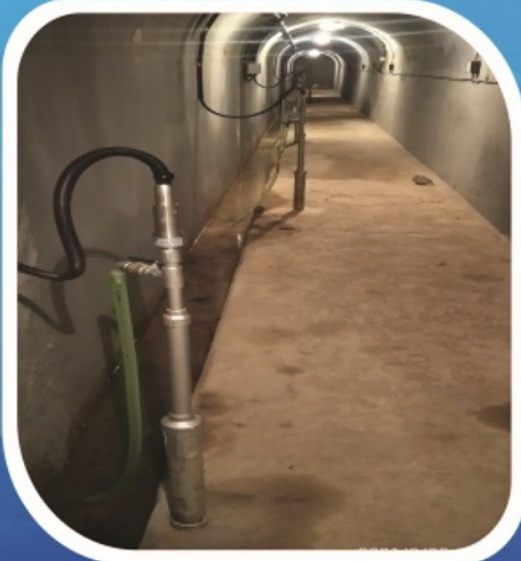
Up-lift Pressure gauge
