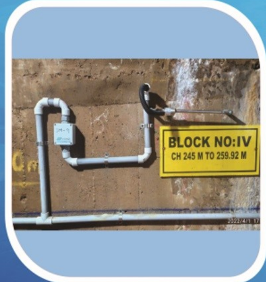
Joint / Crack meter
